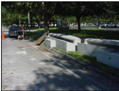
Uninstalled Curb Cuts
